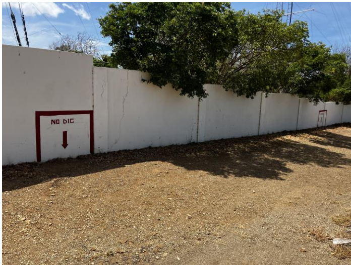
“No Dig” markings
