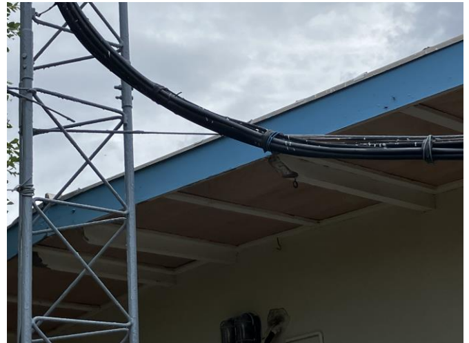
The tower end of the new messenger showing grey epoxy coated dead end and attachment point.
