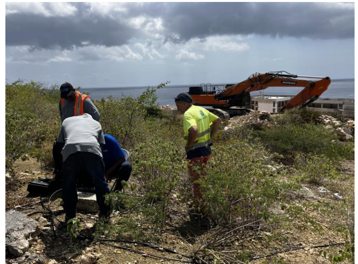
Testing a fibre splice box on the Ridge while an amazed heavy equipment operator looks on. February 12.
