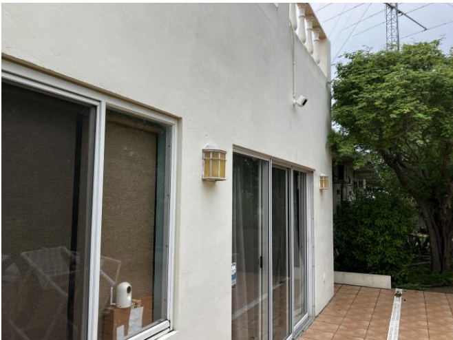
New Ring camera above sliding doors that provides continuous surveillance of the generator.
