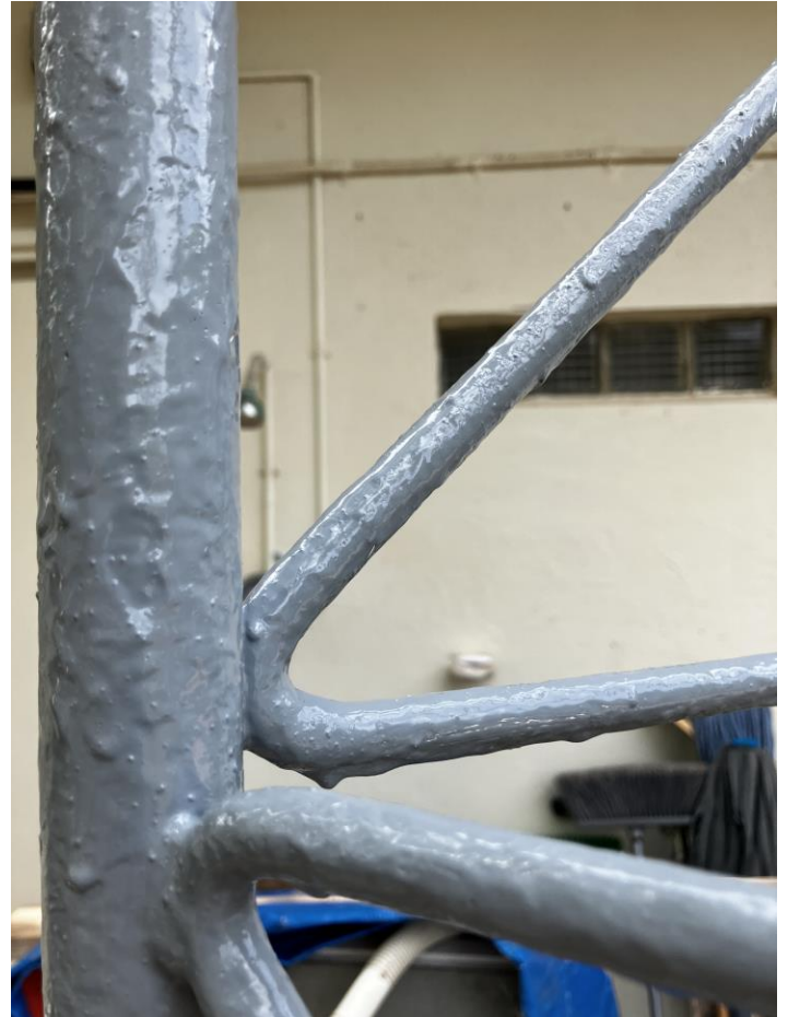
Close-up of the super new epoxy finish at the bottom of the US/JA tower
