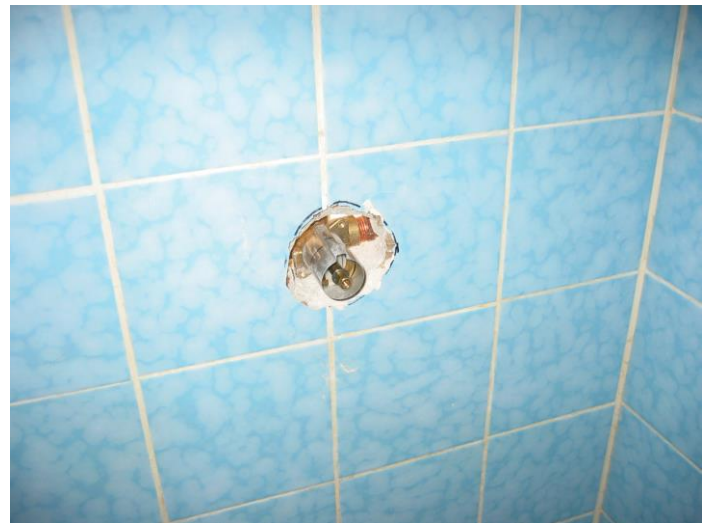
The new assembly inserted into the hole that I laboriously hand chiseled through a 4 inch thick concrete wall.
