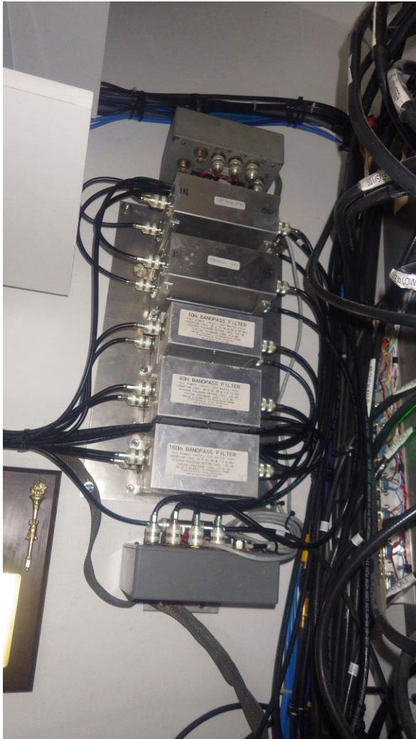
The bank of filters for remote station
