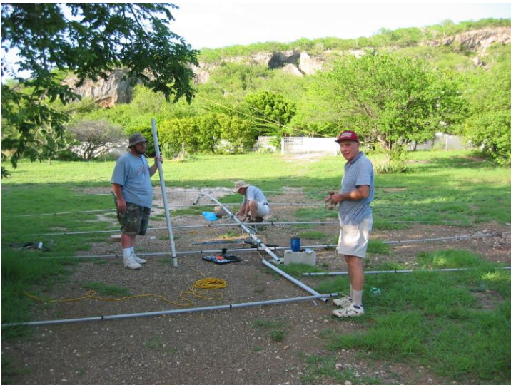
K8ND joins in as we reassemble the rehabilitated antenna. Since this rebuild it has been trouble-free.
