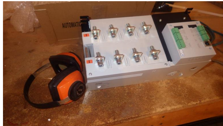
PJ2T's generator AC transfer switch
