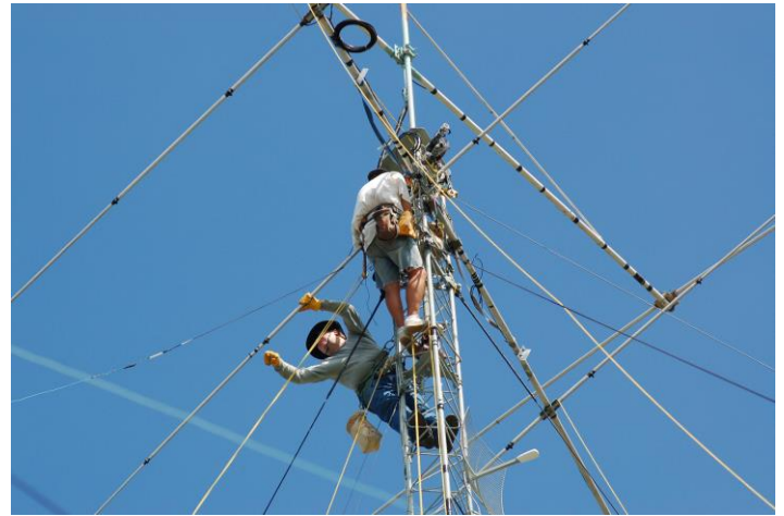
W0CG and W8WTS at 100 feet reinstalling a rebuilt antenna on the Europe tower, November 24, 2006.
