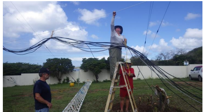
W8WTS rustling a very heavy and unruly bundle of feedlines back onto the messenger cable to the new tower.
