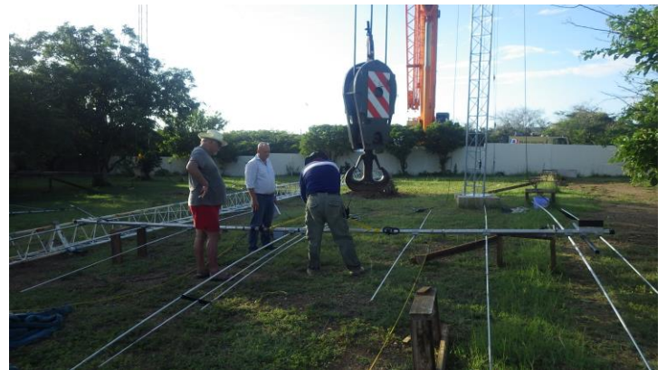
Rigging the Bencher Europe Yard antenna to go up on the crane. We managed to put up two yagis on December 4 before we ran out of time and daylight. We did the rest of the installs the next day using Armstrong methodology, with VE3CX serving as the Human Winch.
