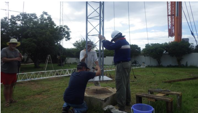
Hanging from the crane hook 120 feet above us, we're finessing the new tower onto the base bolts. Note the crane boom in the distance at the right.
