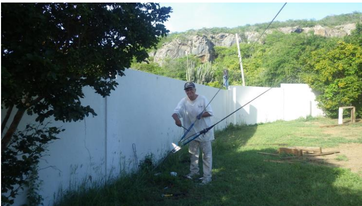
A very relieved W0CG tensioning one set of guys while W8WTS and VE3CX concurrently do the other two sets.
