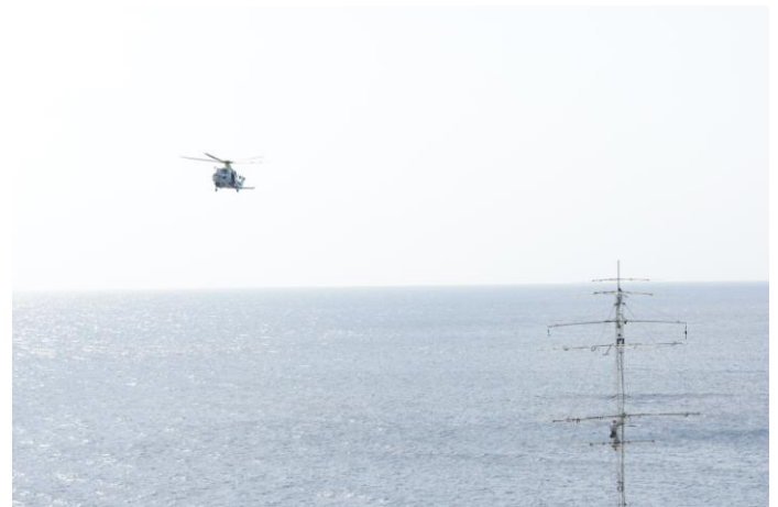
W0CG working on the US/JA tower, February 24, 2024, with the Coast Guard chopper monitoring. They waved! (K8ND drone photo)
