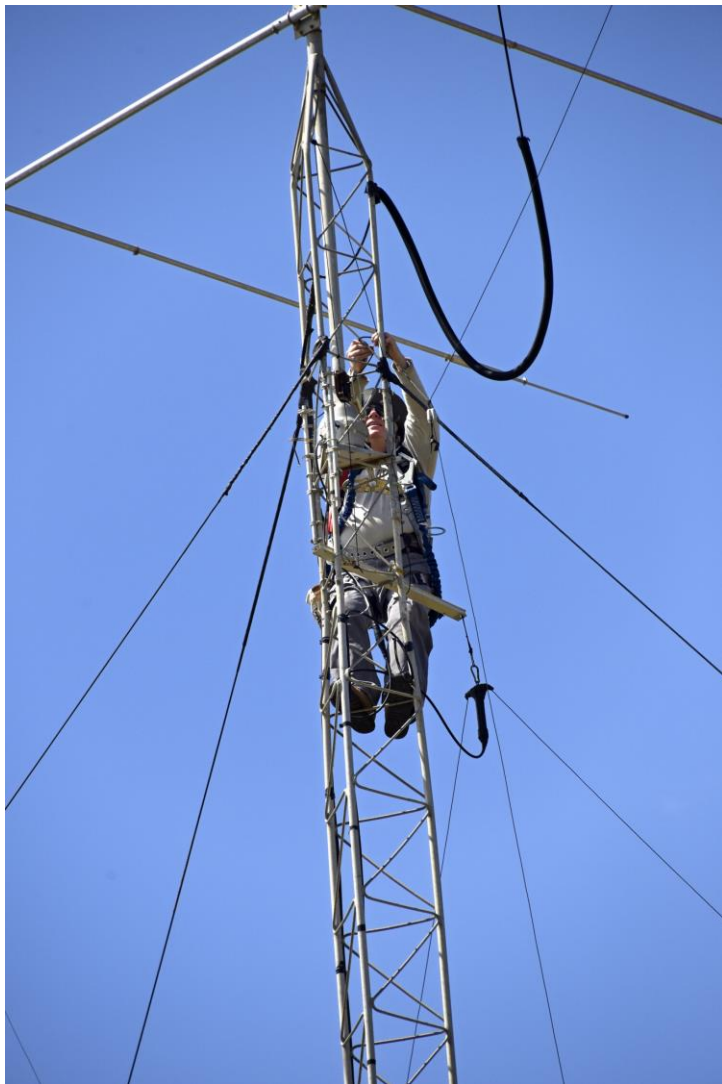
W8WTS near the top of the WARC tower, 55 feet, patiently stringing a replacement rope
