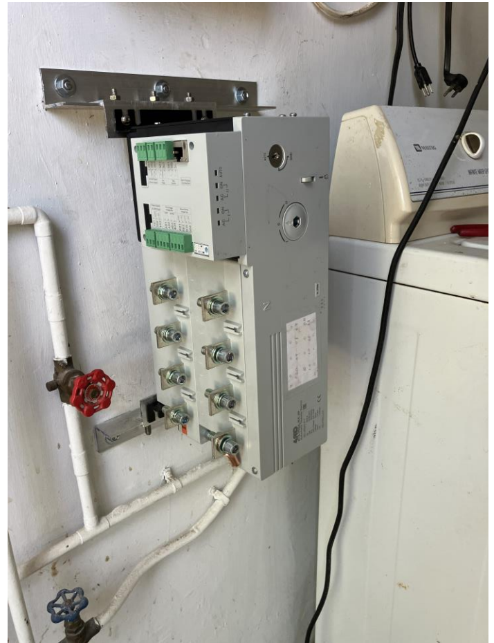
Generator transfer switch installed in utility room
