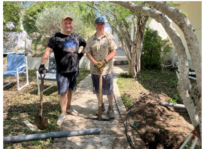
PC8M (Pim) and W7EY (James) taking a break from vicious digging under the sidewalk in blistering heat
