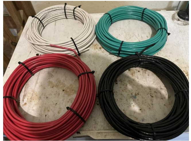
#6 AWG Cu from generator to house, 26 September 2024
