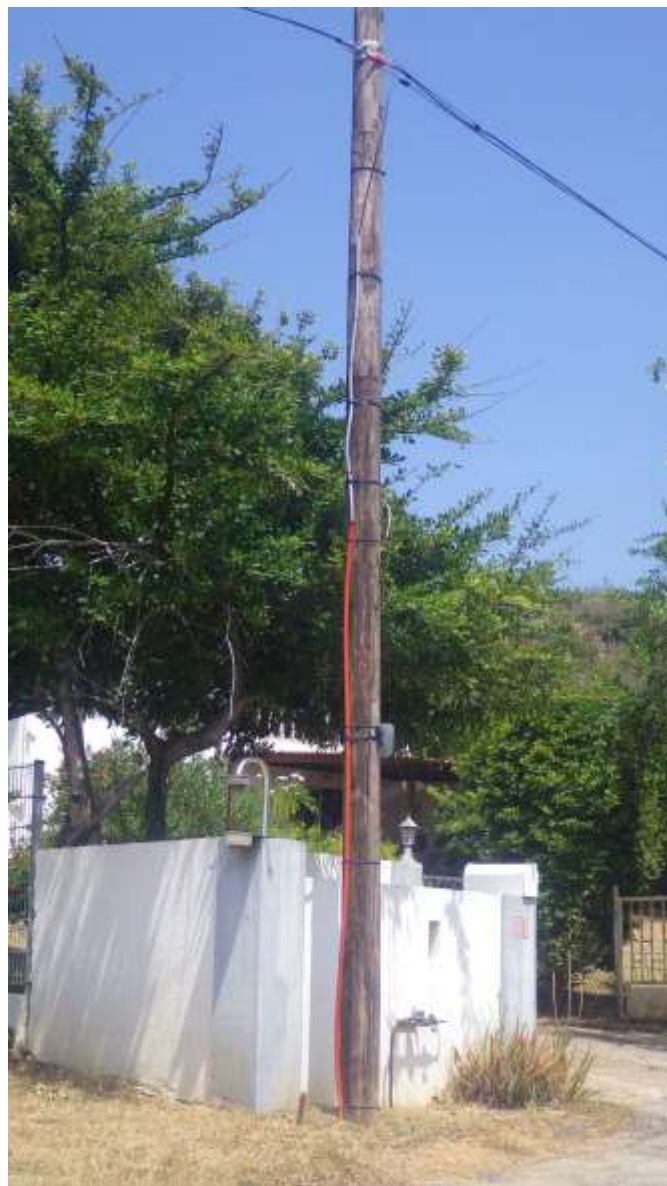
Signal Point fiber (black at the top) protected by grey and orange conduits.
