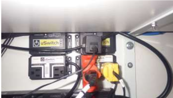
Remote station AC power configuration. The left switch has now been removed for return to the vendor.
