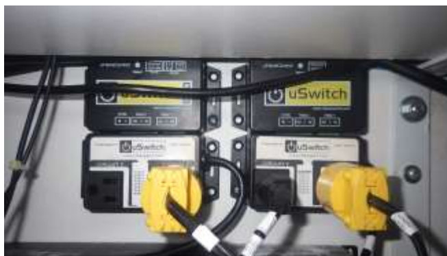
Port 72 and Port 73 remote AC control switches
