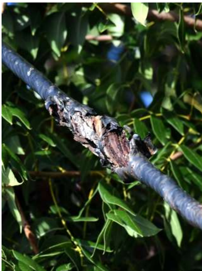
Damaged guy wire waterproofing from tree abrasion
