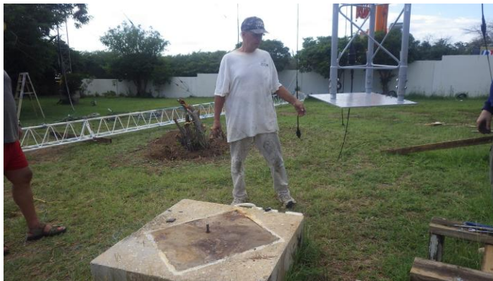
W0CG as the new tower, hanging on the crane 120 feet above, nears touchdown.
