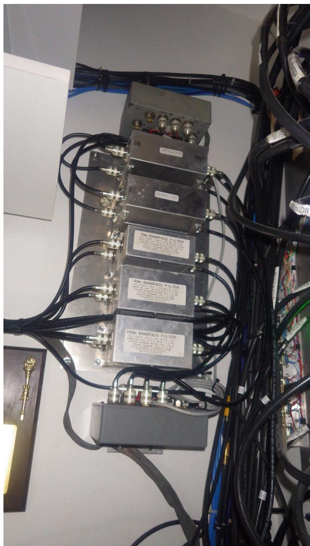
Remote station bandpass filter bank
