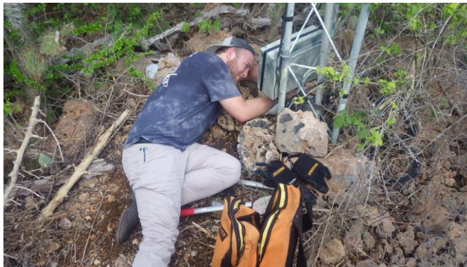
Levi, KG5XR, reconnecting cables after reinstalling the coax switch box at the Ridge tower.
