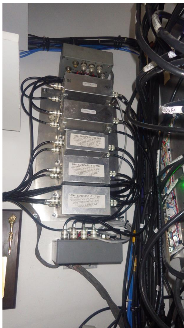
Above and below this filter chassis, built by W8WTS, you can see two 1 x 6 coax switches. These were at PJ2T for many years in surplus and are now in service at the remote station.
