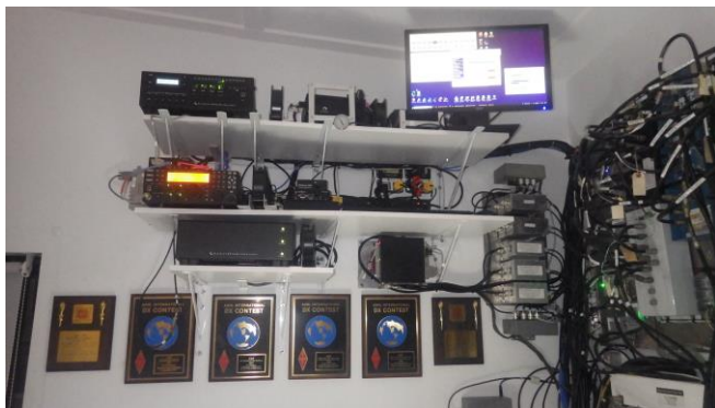
The new block of 10 bandpass filters is at the right, below the monitor. The Bandmaster chassis and two of
