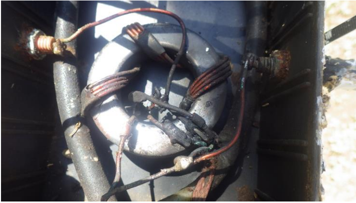
The blasted 160 TX unun transformer on Saturday, DOA.
