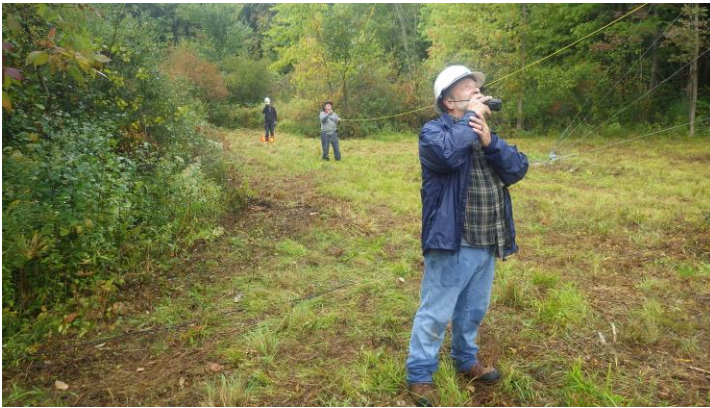
Teamwork: W3YQ managing the climber and crane operator, W8WTS wrangling both tag lines on a monster yagi, and AF8A feeding rope to Jim.
