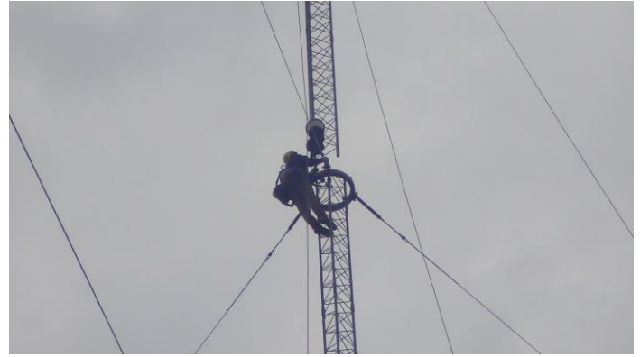
Trevor at about 130 feet ready to connect the top section. Quite a chore for a guy working alone in the rain.
