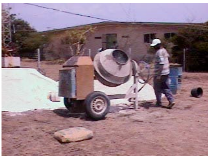
July 2001, mixing concrete for tower bases. Note that there are no Rohn towers and there is no perimeter wall at this stage.
