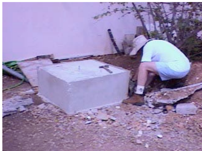
W0NB removing concrete forms from the base of the US/JA tower, July, 2001.
