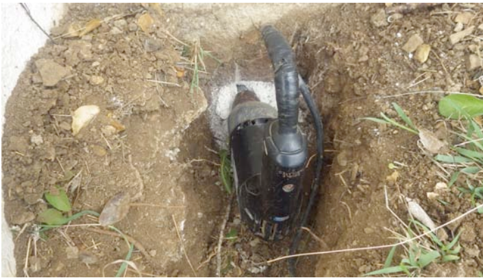
It's through: the bit cut a hole through the 10 inch wall and concrete footer, July 13, 2022.
