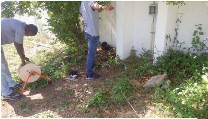
Sorting out the fiber and three pull ropes inside our front wall
