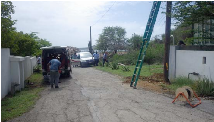
Some of the gaggle of people and vehicles that arrived all at once to install the fiber July 18, 2022.
