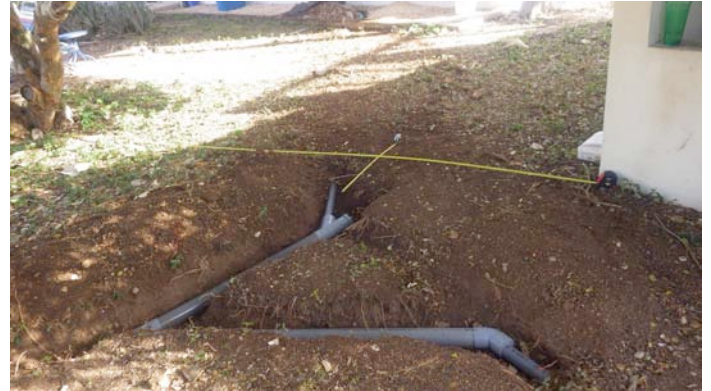
The 50 mm conduit from the road splits here and reduces to two 25 mm branches to the houses. March, before burial.
