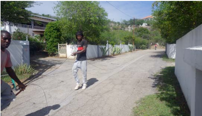
Laying out the fiber to the distant pole, which has the optical splitter box, to be sure we had the proper length before making a cut.
