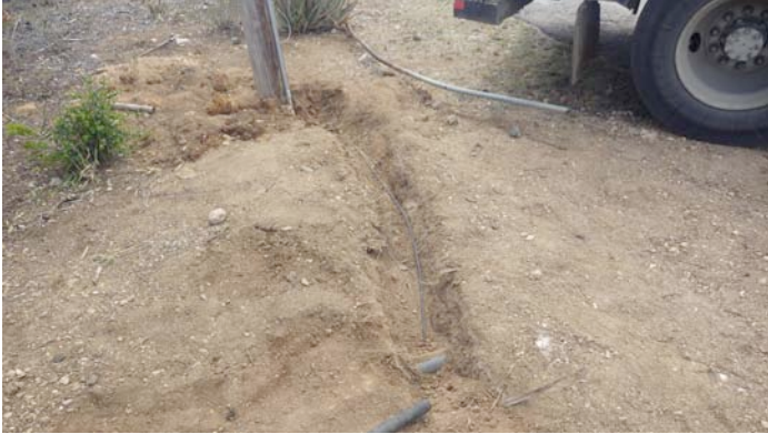
Fiber laid in the ditch, with our grey PJ2T conduit visible. The fiber runs under our conduit. This will be our permanent data feed to all the houses.
