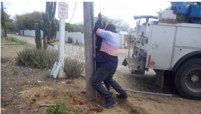
Two guys tugging with all possible might to tension the overhead fiber cable.
