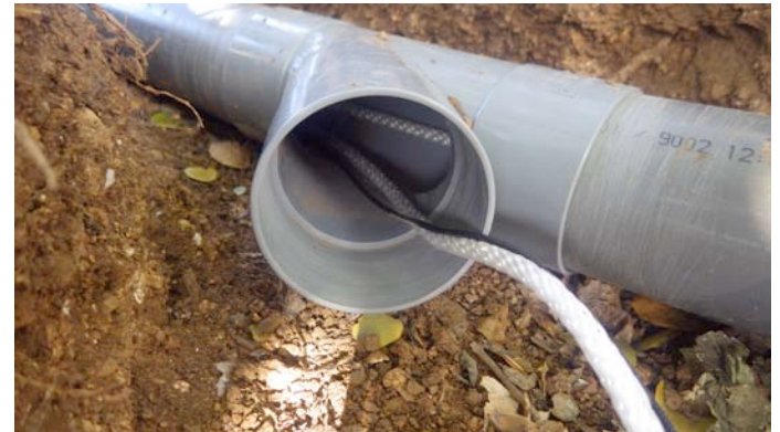
The junction in the buried conduit where the 50 mm tubing takes off for Signal Point.
