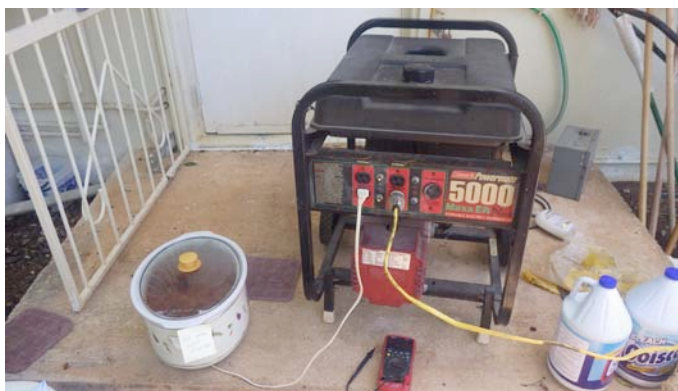
The old 5 KW camping generator keeping PJ2T on the air and the crock pot cooking the chili most of Saturday afternoon.
