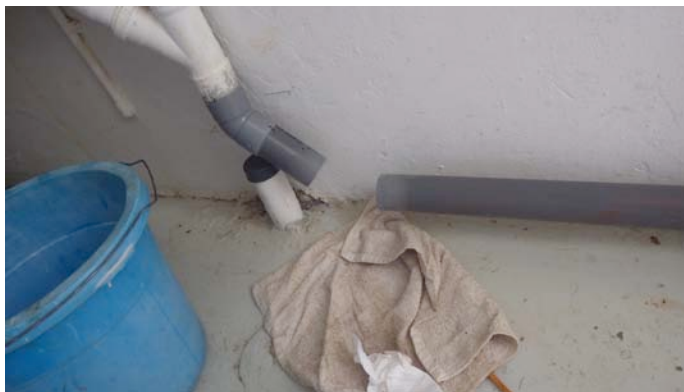
A 45 degree fitting to intercept bathroom sink water and send it outside.
