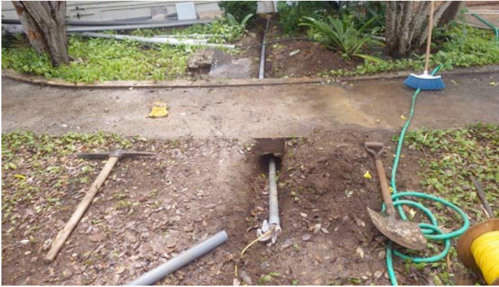
Two days of sloppy muddy work to get this route under the sidewalk for the fibre.
