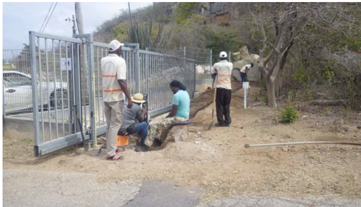
Installing temporary phone line to the neighborhood. Note the white PJ2T RX antenna box.
