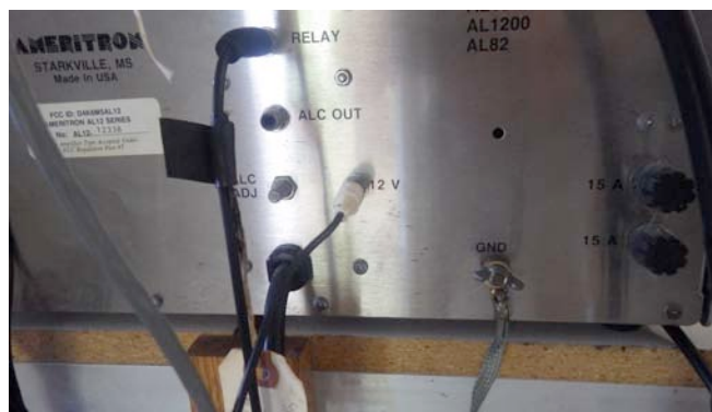
Switched 12 VDC at the back of each AL-1200
