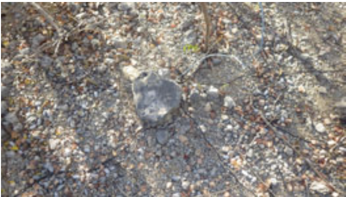
Original termination ground and resistor system at the 880 foot point still in good condition.
