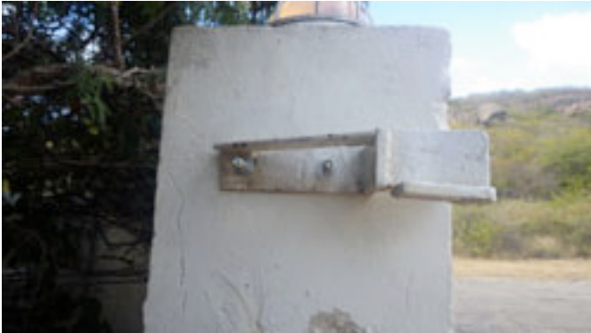
Front gate stop bracket, reinstalled on February 10 for hopefully many years of service.
