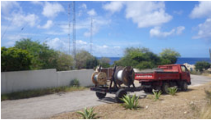
Cable literally at PJ2T's front gate February 10.
