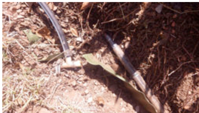
One of several buried junctions opened while searching for the blockage.
