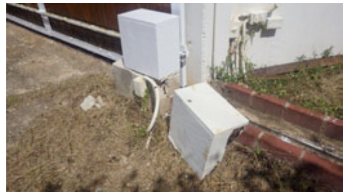
New box in place, sporting two coats of epoxy paint, with the retired rotted box at the right.
