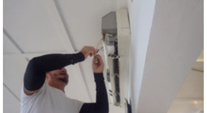
Jack Biscayne patching together the mouse-destroyed wiring to the swing motor, February 12.
