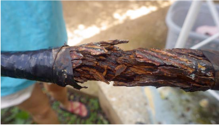
Guy grip about 75% failed on the US/JA tower
