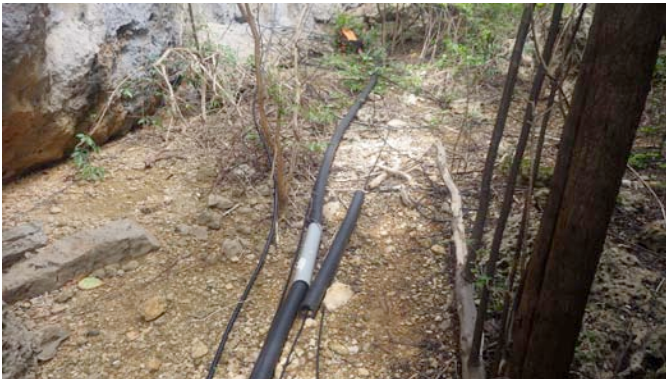
Important PJ2T cabling in the wilderness
