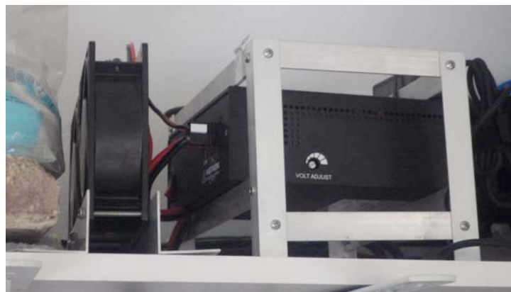
Cooling rack for the DC supply
