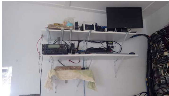
PJ2T's enhanced remote station
