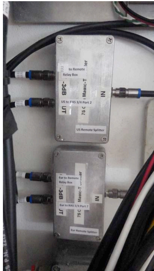
N7IR RX splitter boxes for the remote station
