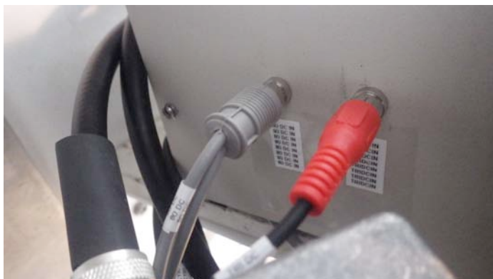
DC control inputs to the NJY Ridge selection box
