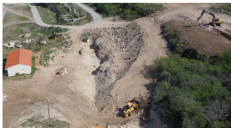
The huge mountain of hotel debris has been reduced to a small hill of concrete with much rebar.
