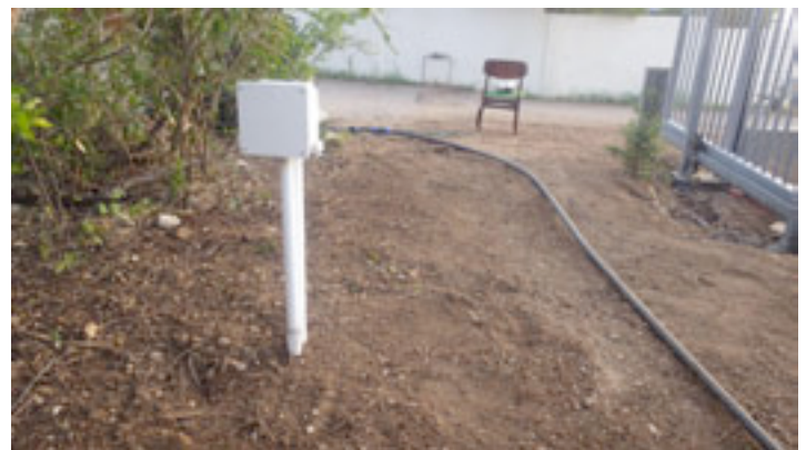
RX antenna feedline box across the road
