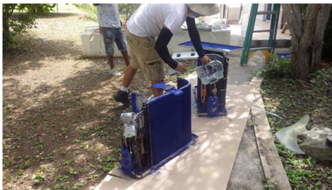
The new 12,000 and 24,000 BTU compressor units drying on the sidewalk, fully coated inside.
