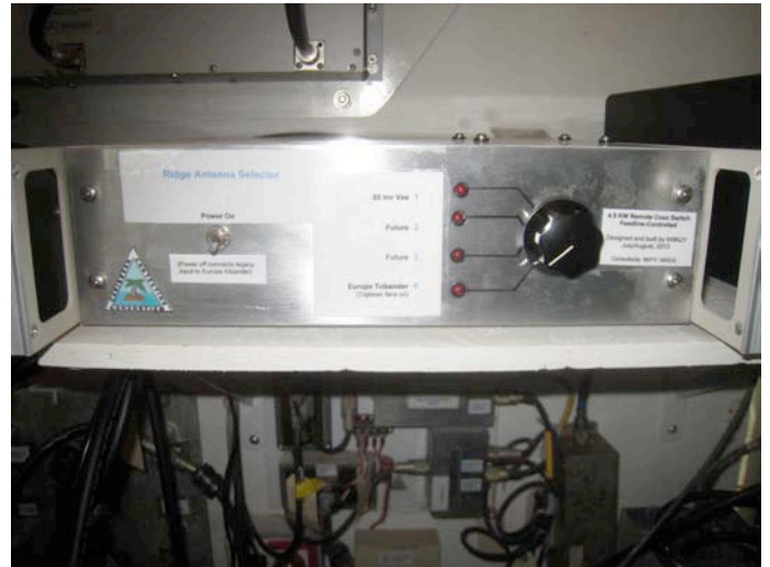
The W9NJY remote coax switch control box in place at Signal Point.
