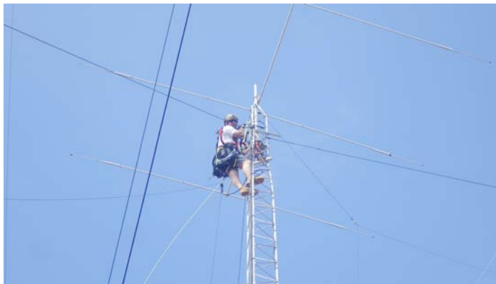
Jason removing the WARC rotor with an angle grinder and a lot of sparks.
