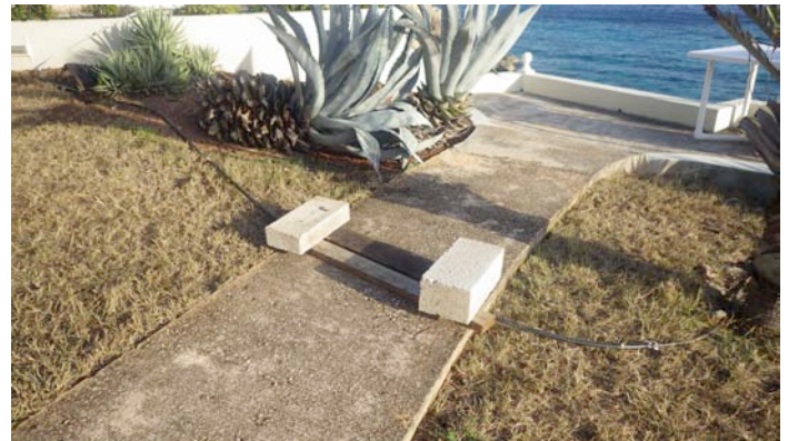
Temporary fix for irrigation problem.
