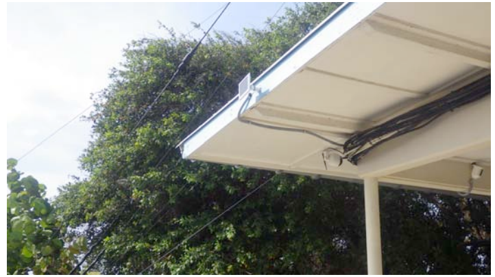
2 watt solar panel that powers the West Porch Ring.
