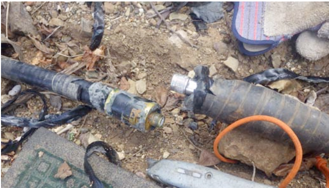
Junction in the Heliac, ready to be reconnected.
