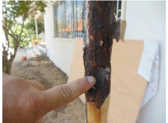
A finger-sized hole in the Ringo Ranger steel mast, March 27, 2013.
