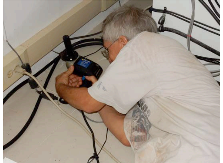
Installing anchors in the masonry wall under the lamp table by the love seat. (K8ND photo)
